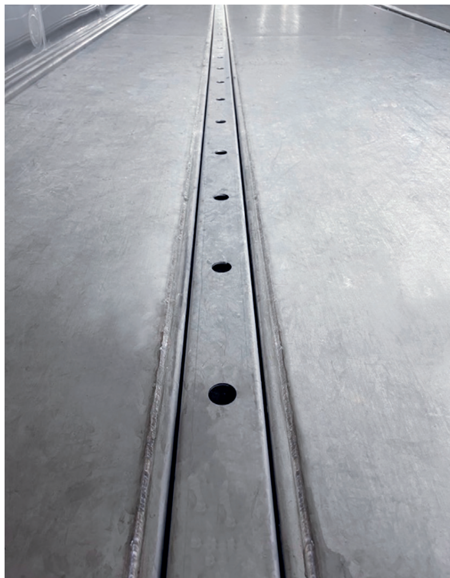
— DRAINAGE CHANNEL running along the middle of the floor under the wagon with cover for easy cleaning
